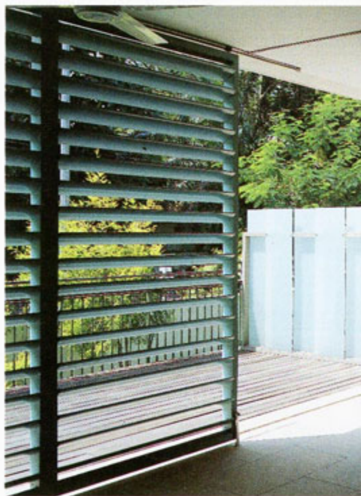
Typical apartment verandah designed as an extension of the living room space (above). Mobile shutters and adjustable louvres give shade and act as a rainscreen.
